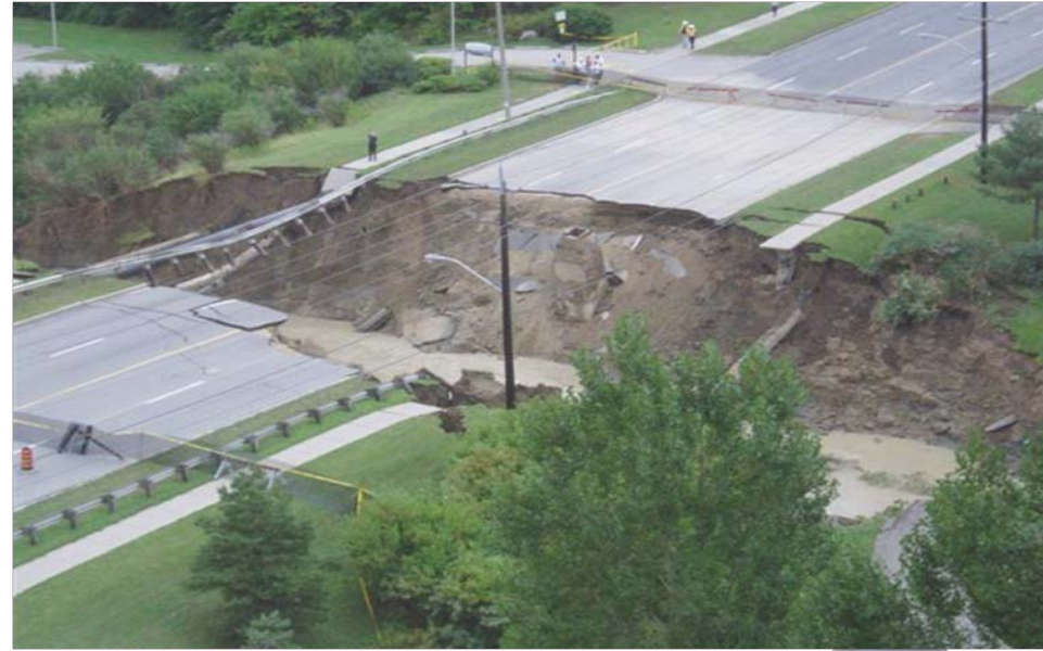
Finch Avenue Collapse, August 19, 2005
